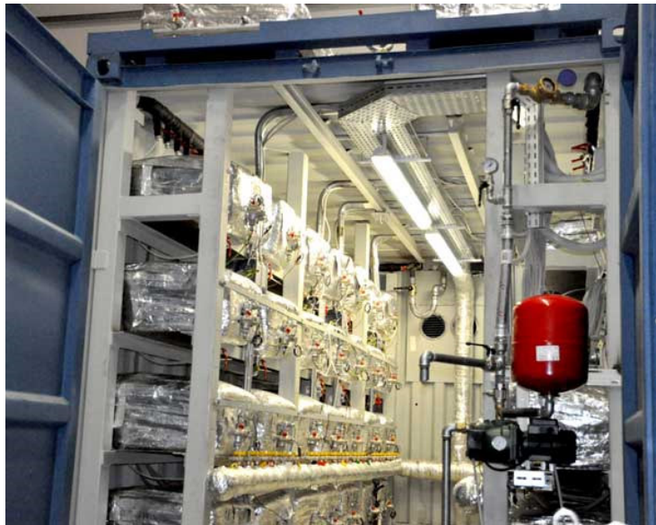
Interior view of the first-generation 1 MW ECAT power plant. Note that the racks are built of smaller ECAT units in parallel.
